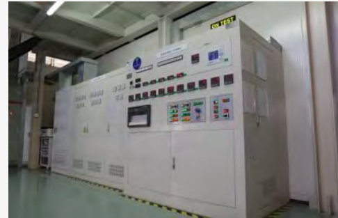
Bus AC Performance Test Room
