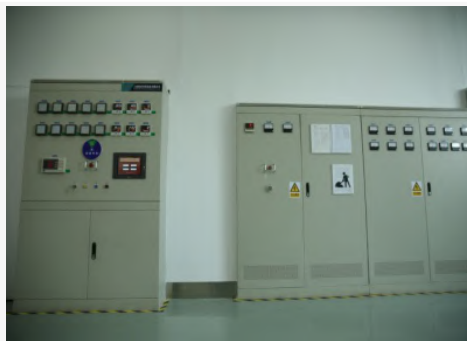
Railway AC Performance Test Room
