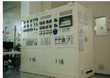
CAR AC Performance Test Room
