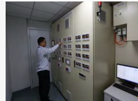
EV Thermal Management Test
